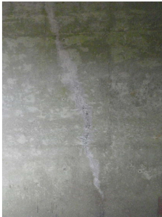
Photo 22: Hairline Crack, typical
