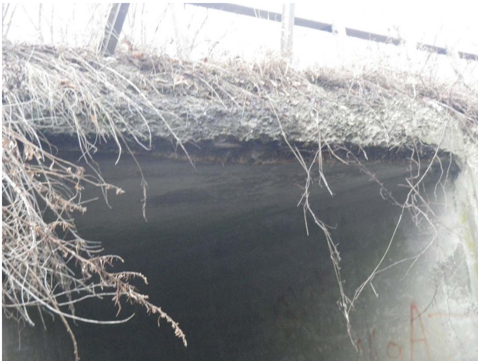
Photo 14: Exposed Rebar, West Fascia Top Slab
