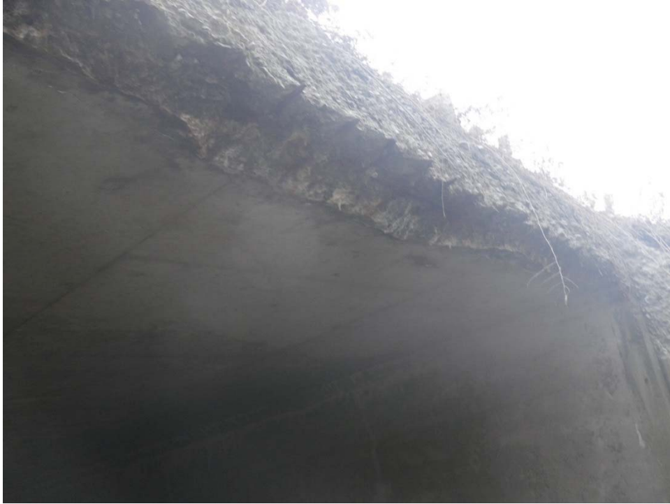
Photo 15: Exposed Rebar, East Fascia Top Slab
