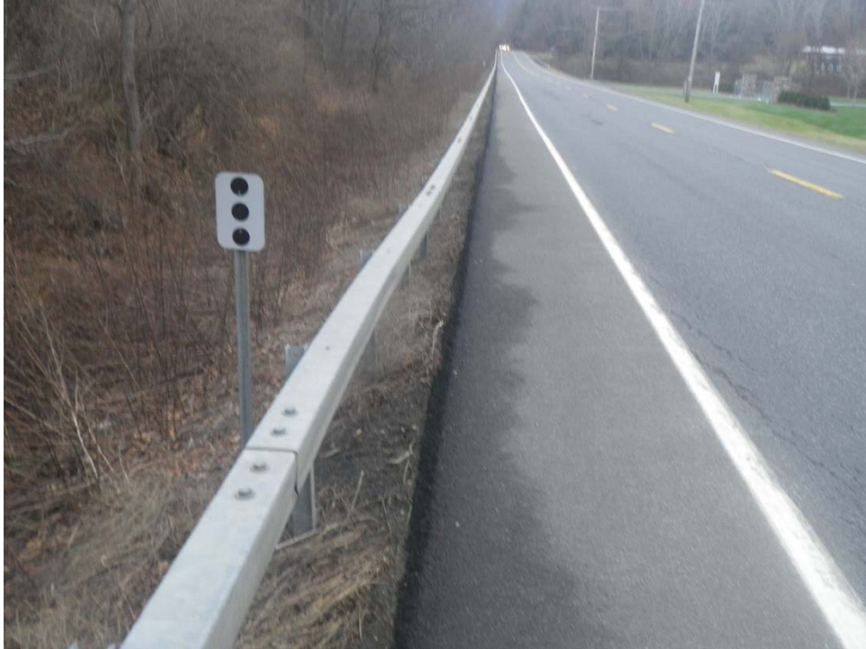
Photo 6: East Bridge Rail, Minor Damage
